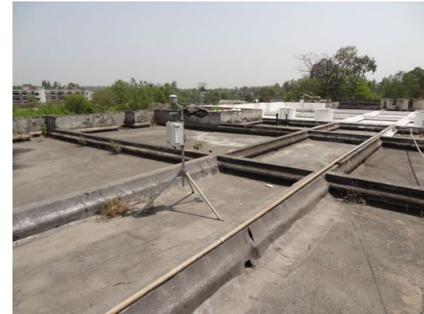
Data monitoring on dark roof
