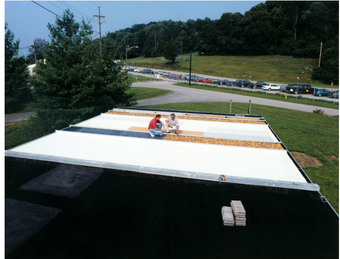
Figure 1 Single-ply membranes were mechanically attached to the ESRA and field tested for three years.
