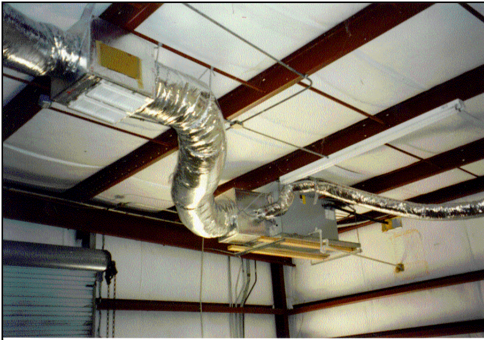
Figure 2. View of roof plenum showing R-11 batts on purlins separated by metal studs with air handler and thermal distribution system located inside the plenum. Acoustic ceiling tiles are typically suspended on the metal frame just below the air handler.
